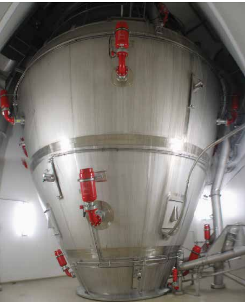
Large volume spray drier protected by an array of explosion suppressors
